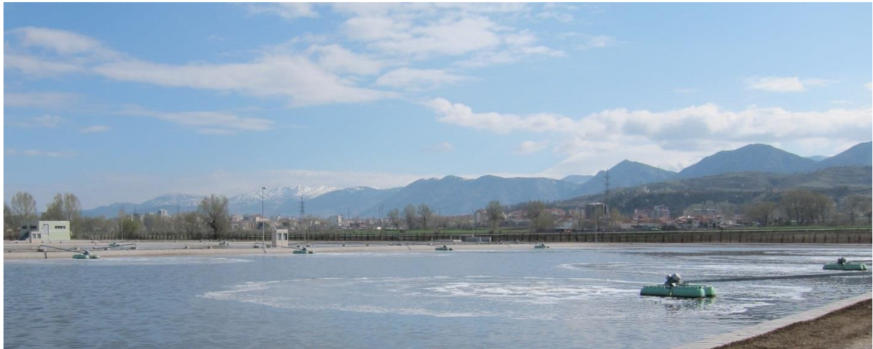
WWTP Korça – Aerated Lagoon System
