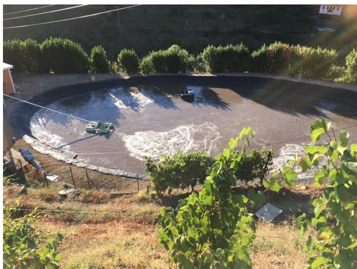
A smaller winery's effluent treatment plant
