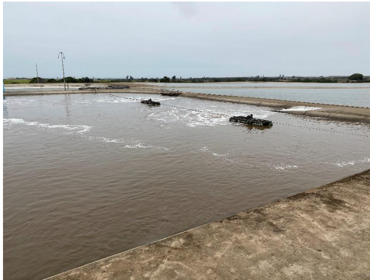
Fig. 3 WWTP El Cortijo: Aeration Lagoon N°2 layout with OxyStar® OS30 aerators in operation in 2022
