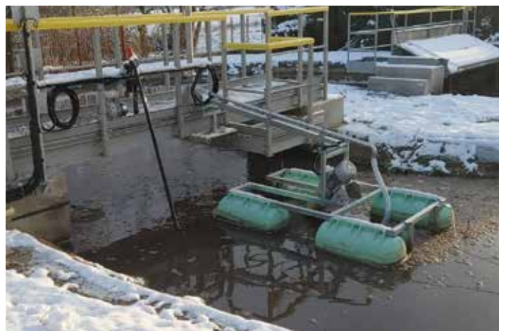
DualStar aerator on floats in a municipal sewage treatment plant (Czech Republic)
