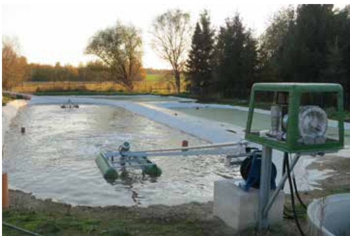
DualStar aerator with a land-side compressor in a sewage treatment plant of a cheese factory (Germany)
