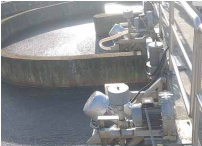
Oxidation ditch of a municipal sewage treatment plant (Czech Republic)
