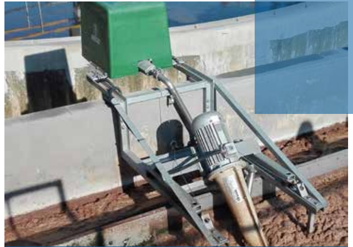
Additional aeration in a sewage treatment plant (France)
