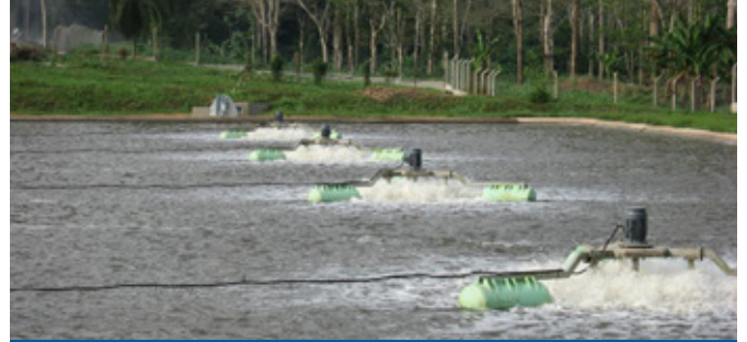
Treatment of wastewater from latex and rubber processing
