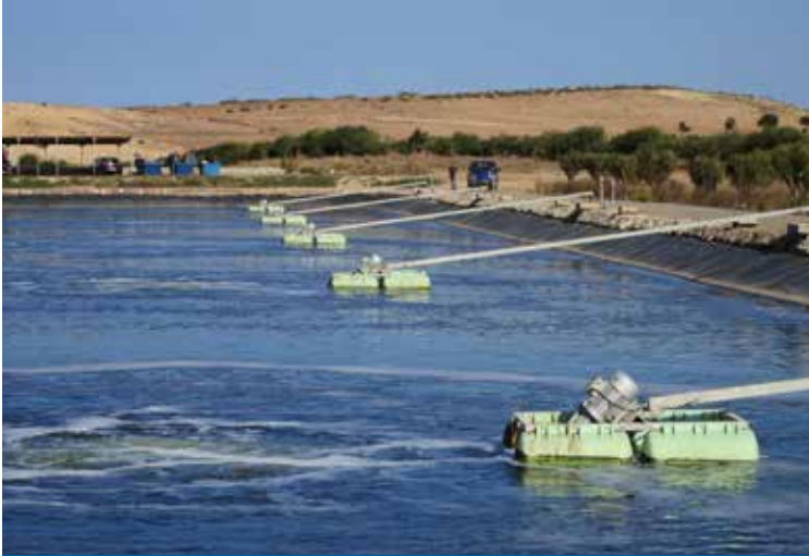
OxyStar® aerators on floats in a wastewater lagoon (Morocco)
