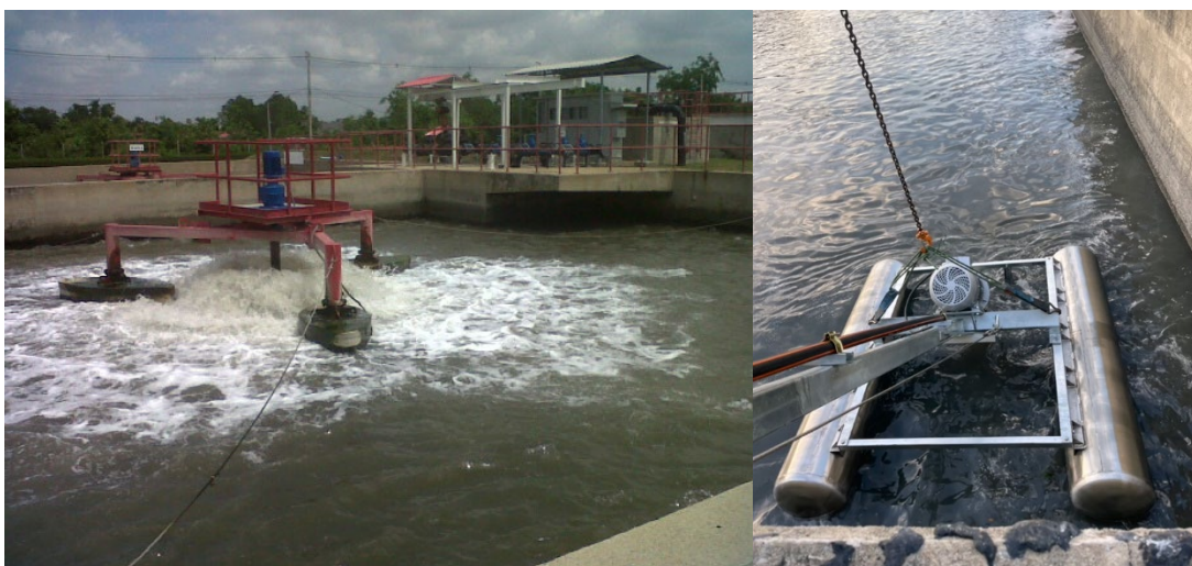
Low-speed surface aerators before replacement (left) and new OxyStar® Aerators during installation (right)!
