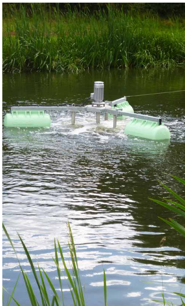
Low-maintenance Centrox pond aerator in a wastewater lagoon
