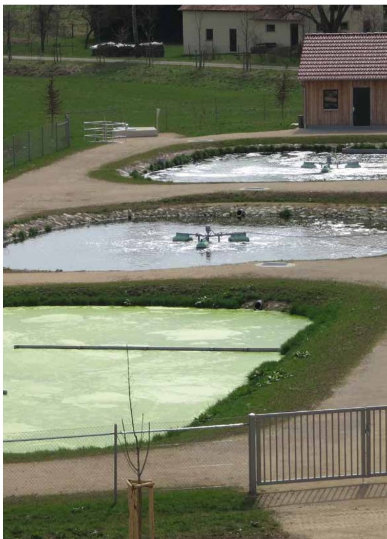
Centrox pond aerators in a small municipal wastewater treatment plant (Germany)
